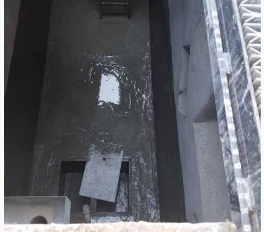
Electric volt in Water table sealed , Brooklyn NY
